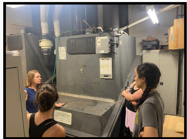
Gathered around a composting toilet system at Thorpewood Learning Center in Thurmont, MD
